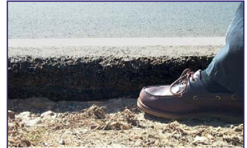
A vertical drop off such as the one shown in this photo is estimated at about 4-5 inches, which is considered a hazard if a driver’s vehicle slips off the pavement and onto an unpaved shoulder.
